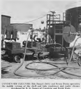
CONDENSER CLEANER: Ildo Donati (left) and Bruno Danis operating the mobile version of the shell and tube condenser and cooler cleaner developed by L. G. Lopez of Catalytic and Light Ends.
